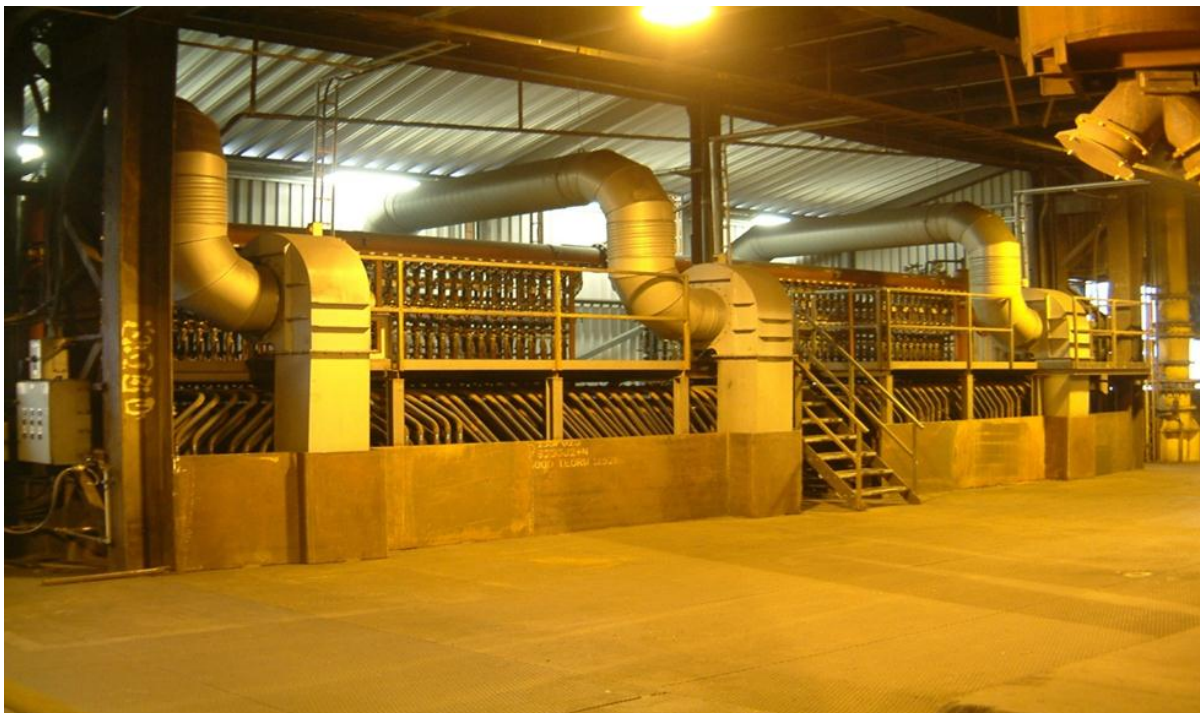
Figure 9: Manifolds for cooling system at Eramet furnace. Ultrasound flow meters are mounted on the inlets and outlets, and water leakages are detected by investigating flow differences.
